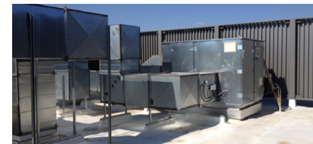
Rooftop installation of RenewAire ERVs at GCU. Image courtesy of MSA Engineering Consultants.
